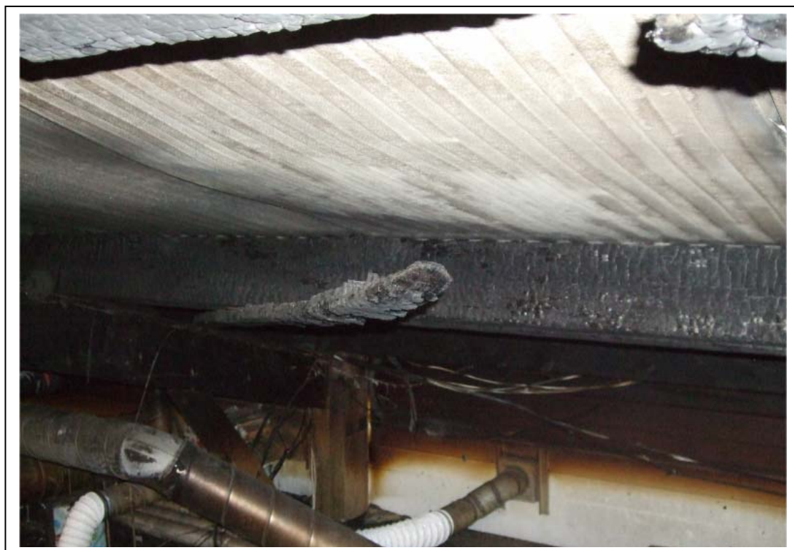
Figure 5 – view of fire damaged area looking down towards the eaves
