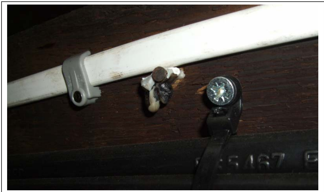
Figure 9 – melted cable clip on smoke stained timber
